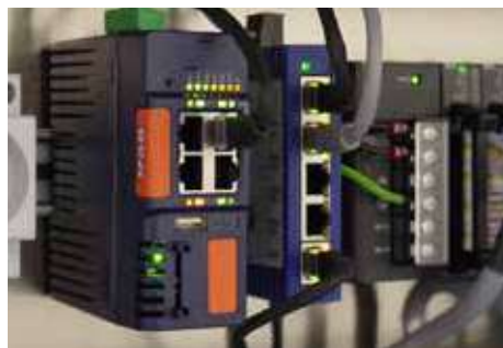
Internet connection for remote maintenance service
